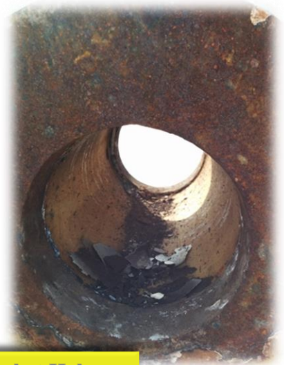
Damage Bracket Hole
